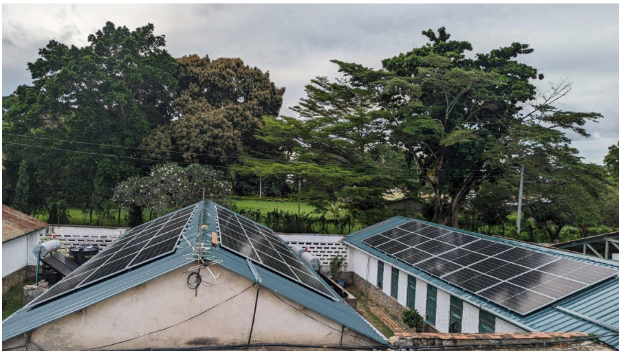
The new solar panels at the APDK clinic in Mombasa
